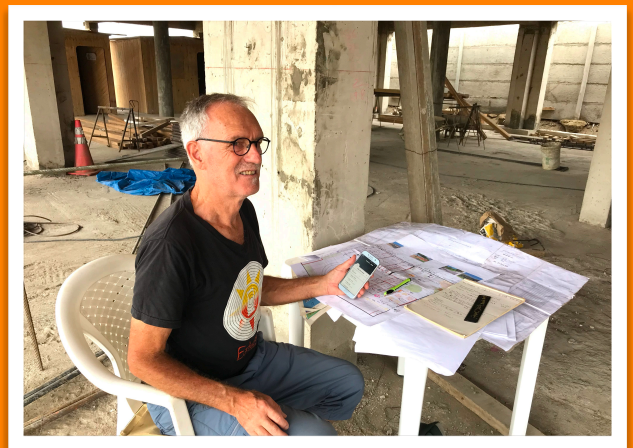
Theo (Swiss construction manager) on the construction site with the construction plans
